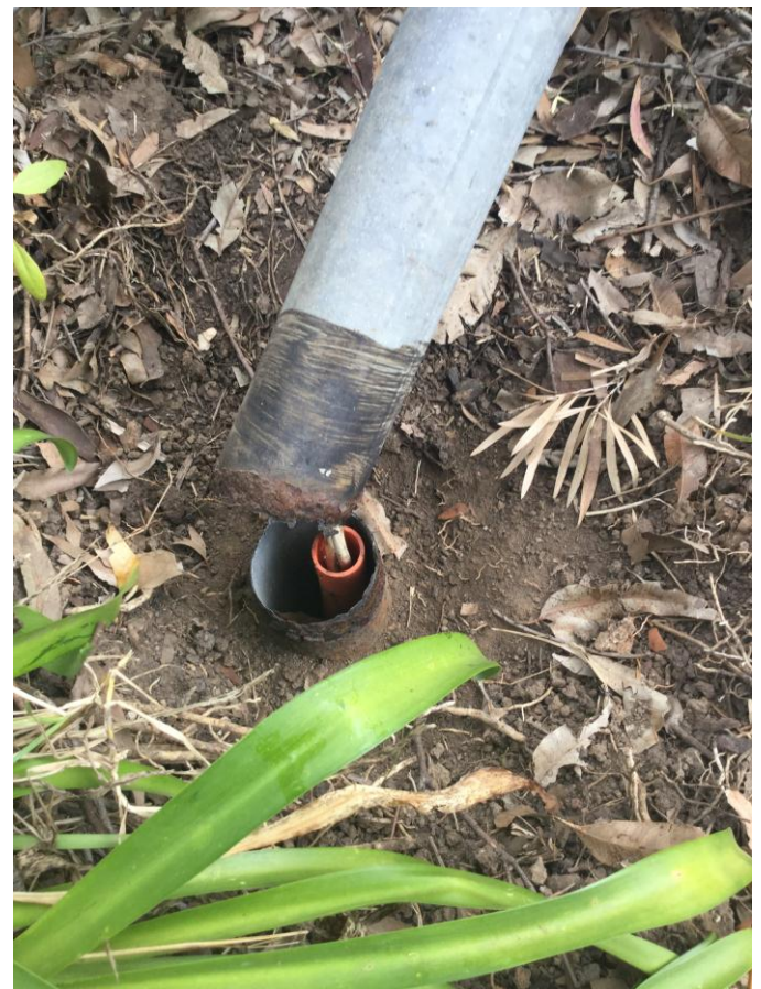
Figure 1. Rusted pole base – pole failure.
