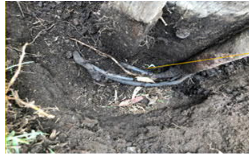
Fig. 1 – Direct buried LV cable damage (at 150mm depth)
