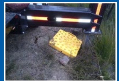
Image of Stabiliser leg and ground subsidence
